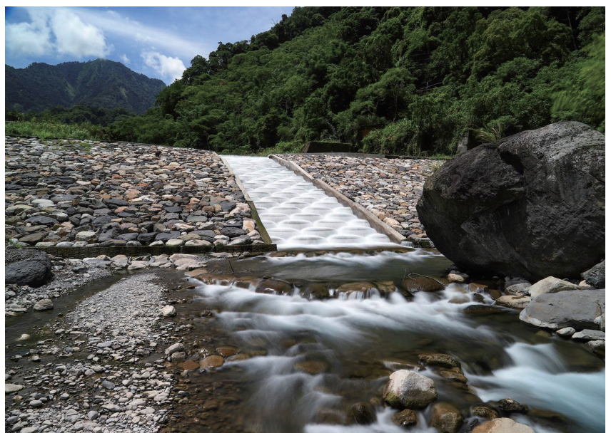
▲ Figure 2-29 Improvement work at a check dam upstream of the Changjung Bridge at Wushikeng River in Taichung
